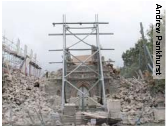
Durham Street Methodist Church, Christchurch, after 22 February 2011.
